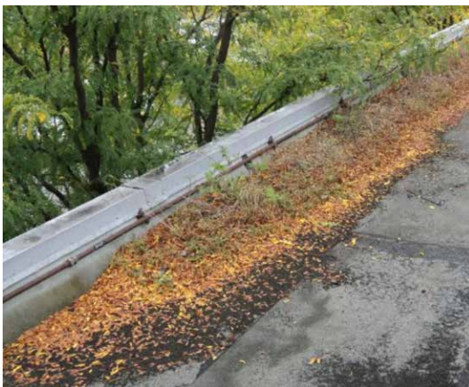
Photo 2. Debris accumulation on the roof edge affecting the effectiveness of the roof surface drainage system [16-S2].
