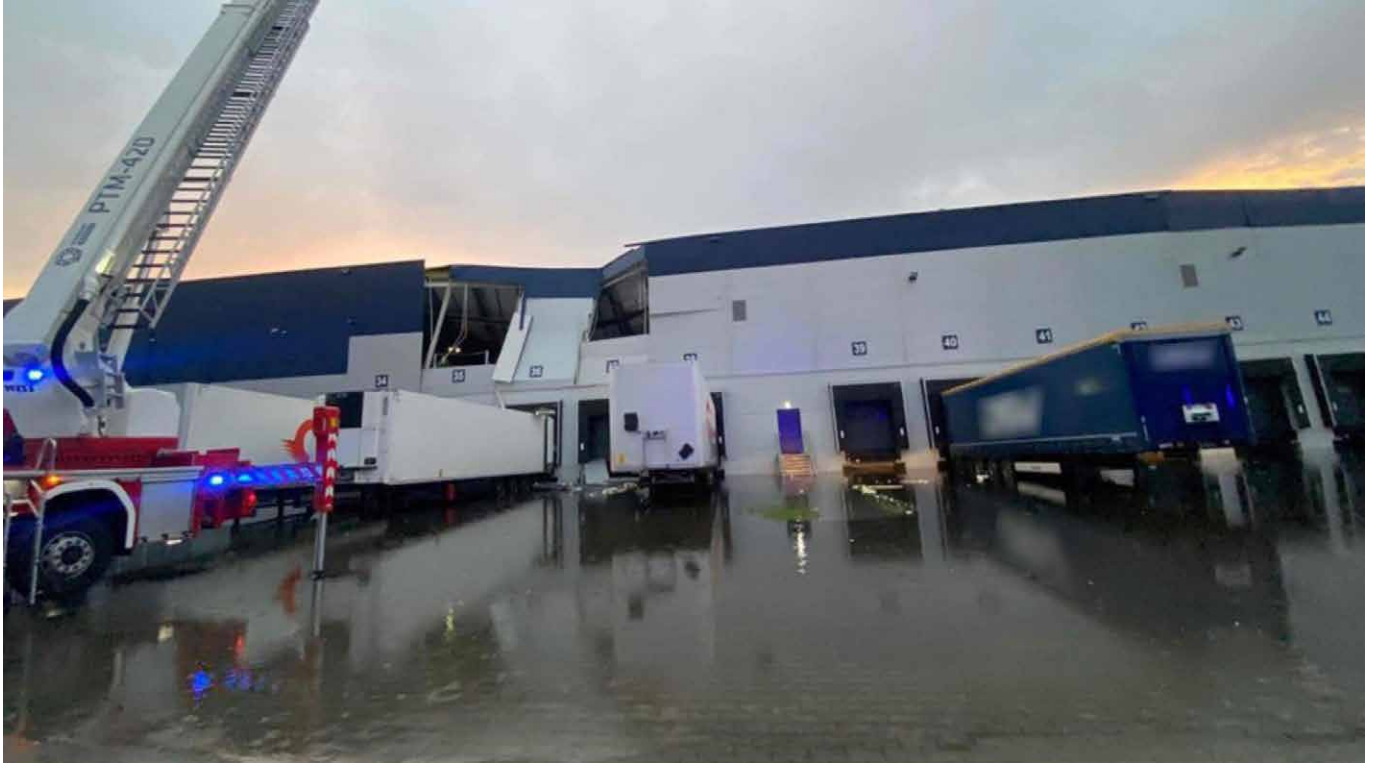
Photo 1. Szczecin. Collapsed roof of the hall at Kablowa Street [S1].
